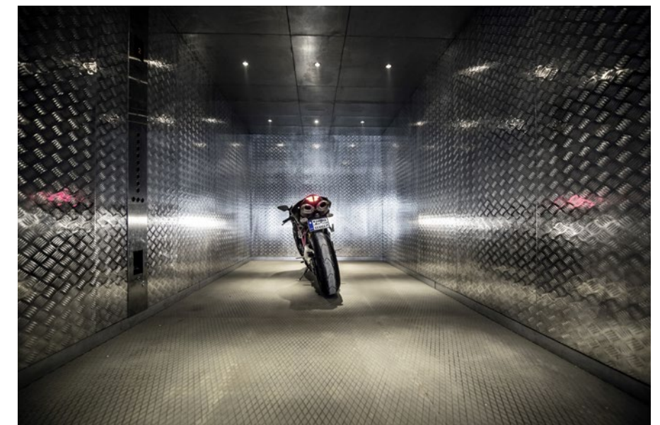
A freight elevator can be used to transport vehicles and other large loads.
